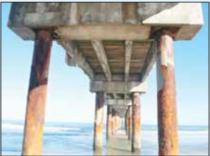
Photo courtesy St. Johns County Support pylons underneath the St. Johns County Ocean and Fishing Pier.
