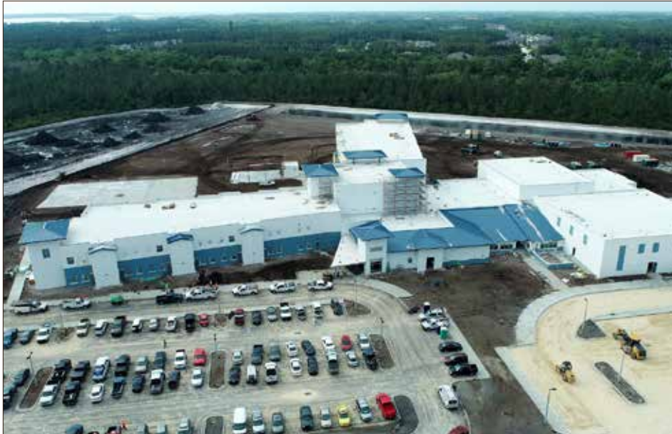
Photo courtesy St. Johns County School District Aerial view of Pine Island Academy under construction as of April 19.
