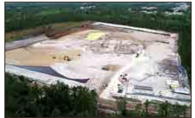
Photo courtesy St. Johns County School District K-8 School MM under construction in May 2020.
