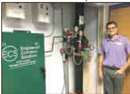
Librarian Chett Wood stands by the new nitrogen fire suppression system.
