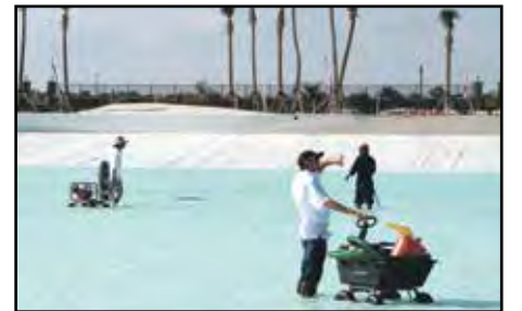
Photo courtesy mbpr group. Workers have begun filling the Crystal Lagoon at Beachwalk.
